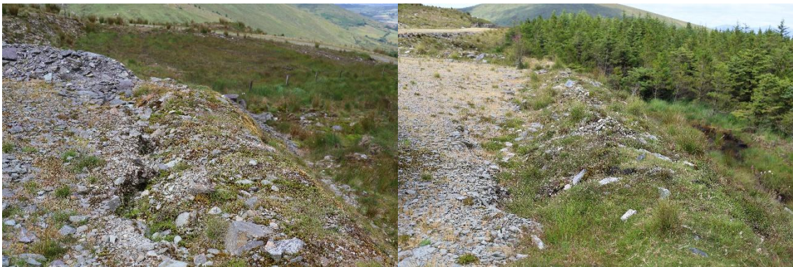
Plate 7.4: Settlement Cracks in Hardstands of Permitted Turbines T02 & T03
